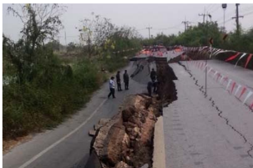
Fig. 1 Road along the canal no.13 collapsed
