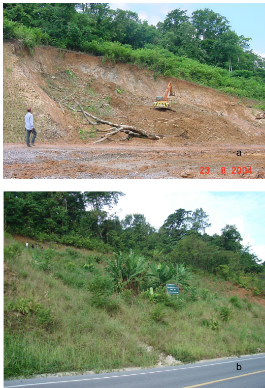
Figure 1 The studied slope (a) in 2004, after failure (b) in current state after regrading and vetiver grassing
