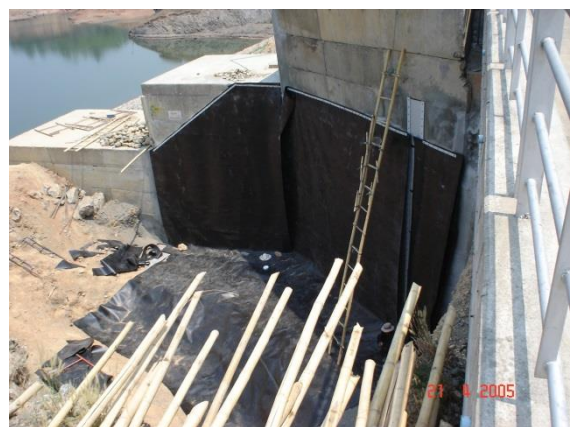
Figure 7 The repair work by installing the impervious membrane over the surface of RCC blocks
