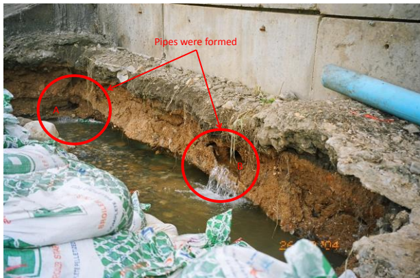
Figure 5 The photos of the leakage
