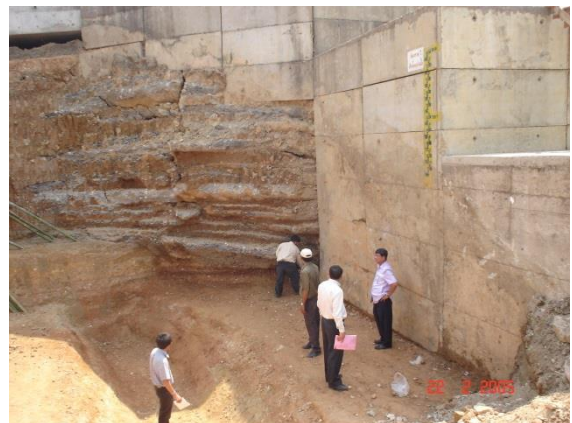
Figure 6 The crack in the RCC block and opening of RCC lift joints
