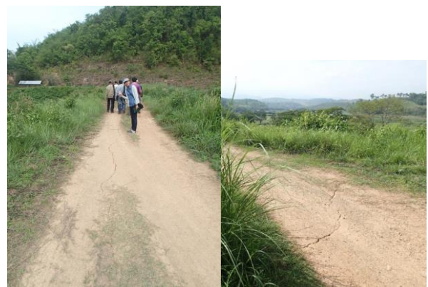
Figure 21 : Small longitudinal and transverse cracks
