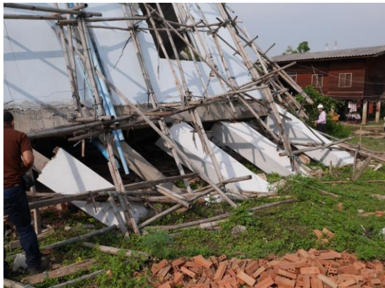
Figure 9 : The damaged of reinforced concrete structure (Picture taken by Dr. Pennung Warnitchai)
