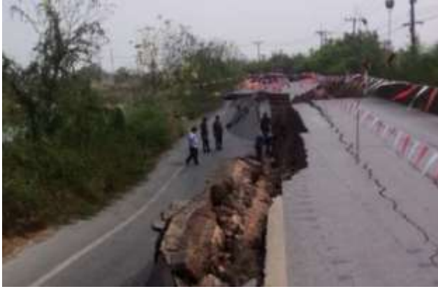
Figure 10: Failure of Road Along the canal (Sasingha & Soralump, 2017)
