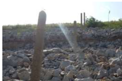
Figure 1: Photograph showing the movement of Pa Bon Dam after first movement
