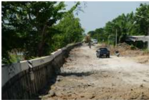
Figure 7 : Failure of embankment along Canal Bank
