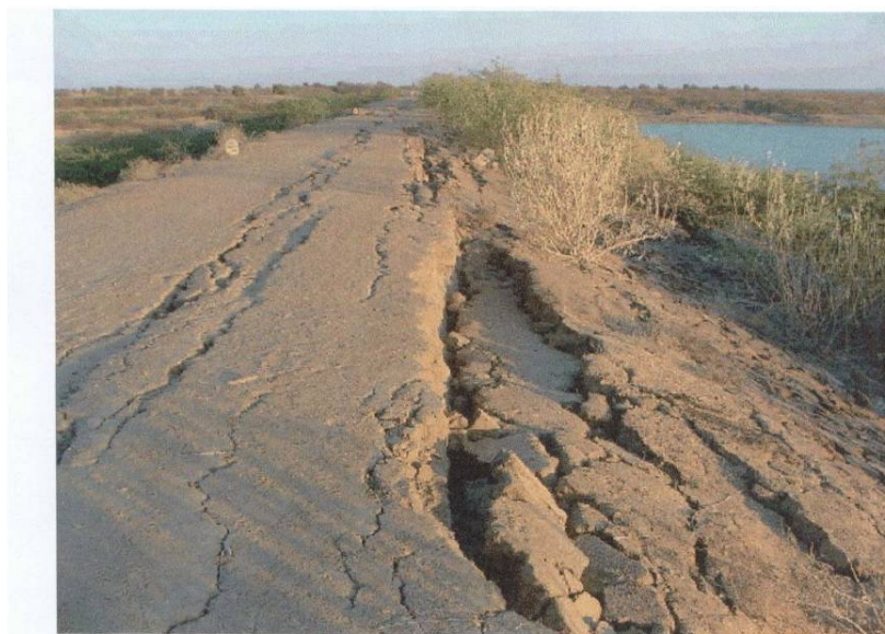
Fig. 2: Longitudinal cracks due to failure of the upstream crest of the Fatehghadh dam caused by the 2001 Bhuj earthquake in India (courtesy Prof. S. K. Jain)
