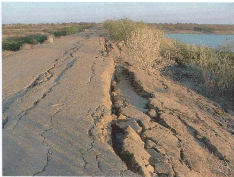
Fig. 2: Longitudinal cracks due to failure of the upstream crest of the Fatehghadh dam caused by the 2001 Bhuj earthquake in India (courtesy Prof. S. K. Jain)
